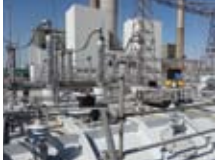
In-situ transformer testing
