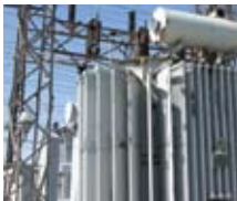
Distribution station equipment
