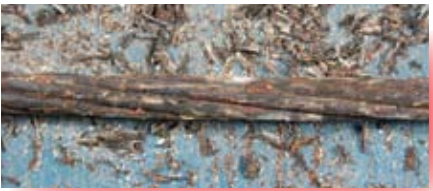
The pictures above indicate the amount of deterioration on the transmission line at the specific distances displayed.
